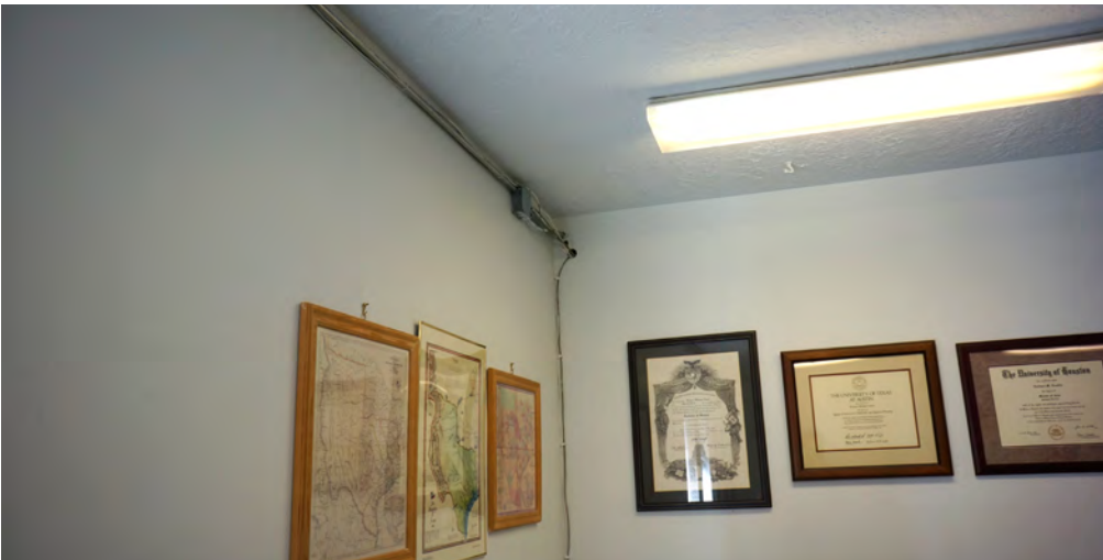
In the City Hall building there are several instances of exposed wiring for lighting, outlets, and boxes.
