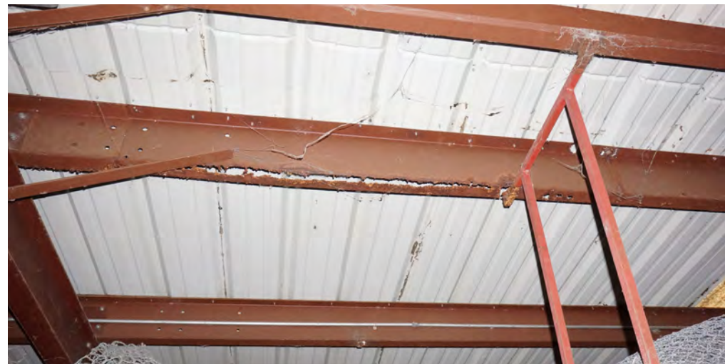
Structural members show signs of major corrosion.
