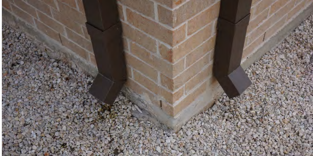
Downspouts on the north side of the building empty directly onto the Police Station’s foundation; this can cause serious foundation issues if not controlled and remediated.
