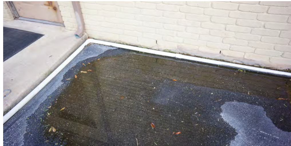
This photo shows the water left from a rain storm at the City Maintenance Staff Building. This illustrates the lack of drainage on the site.
