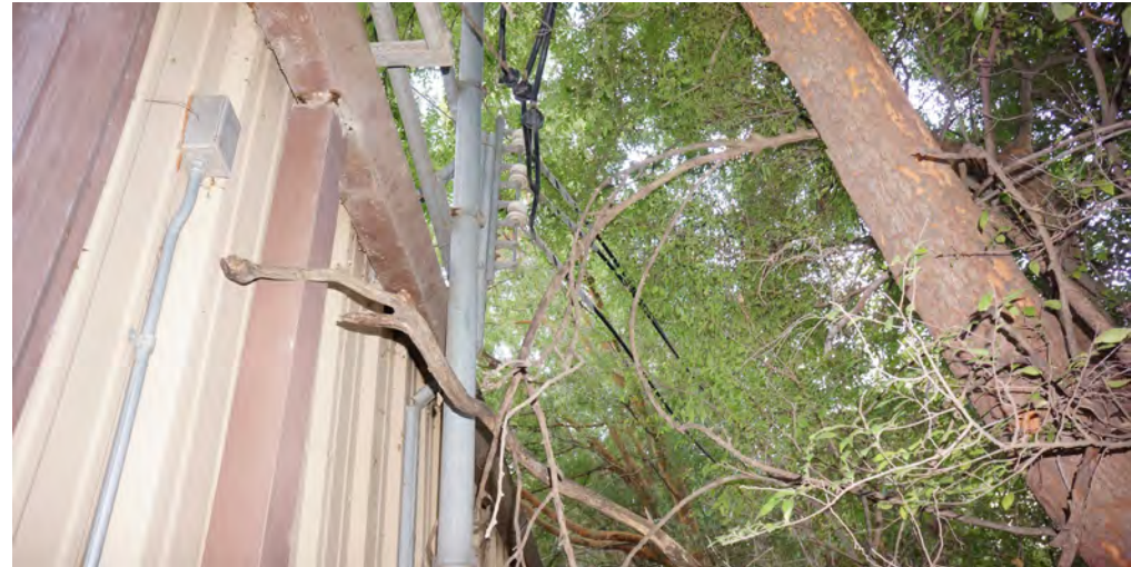
Tree vegetation has grown so much that it interferes with the Golf Course Cart Barn’s power source.
