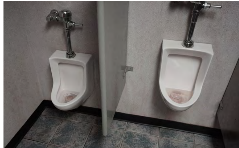
There are faulty plumbing issues throughout the building.
